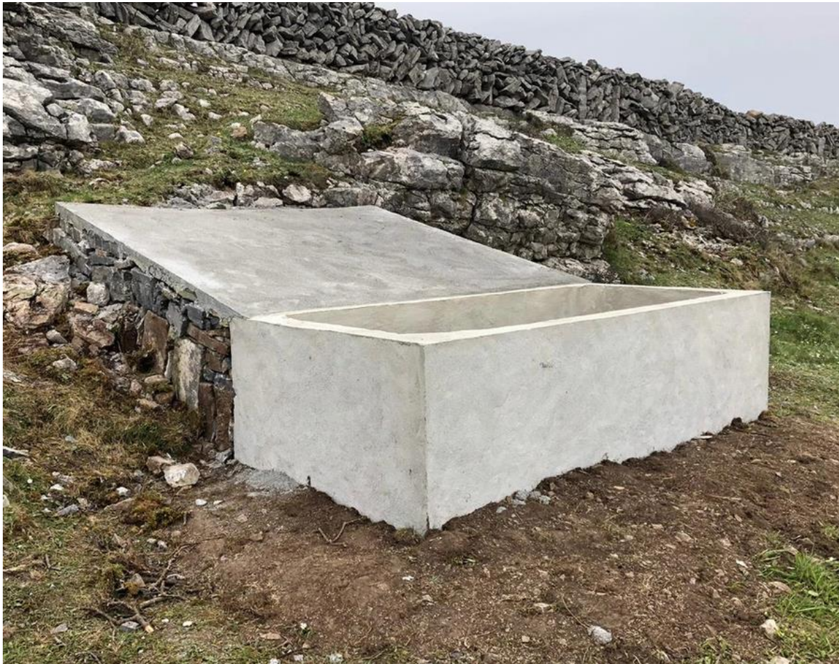
Picture 9: Example of Rainwater Catcher
